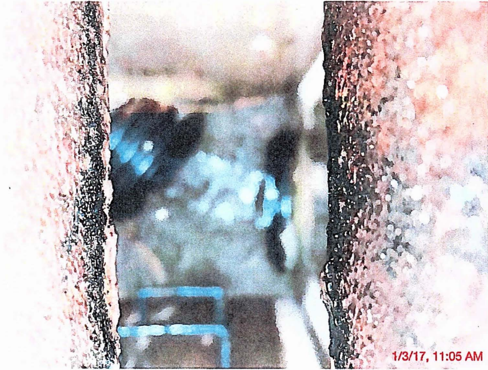
Discharge from JCESA property into storm water basin
